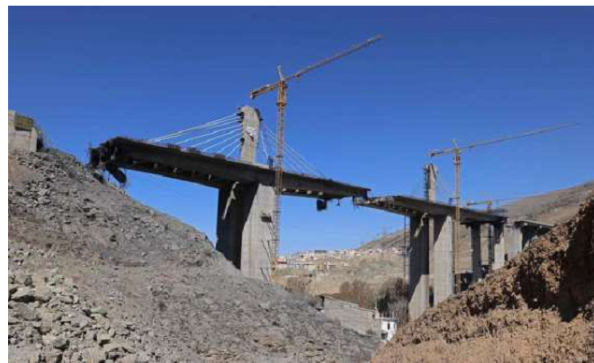
Symbol of resistance: The B1 bridge, after it was destroyed by a strike in Karaj, nearly 35 km southwest of Tehran, on April 3. Donald Trump had previously threatened to bomb Iran 'back to the Stone Ages'. AFP
